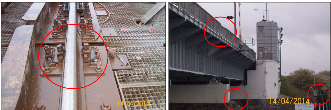
Figure 6: Damage to bridge Source: Rail Net Denmark
